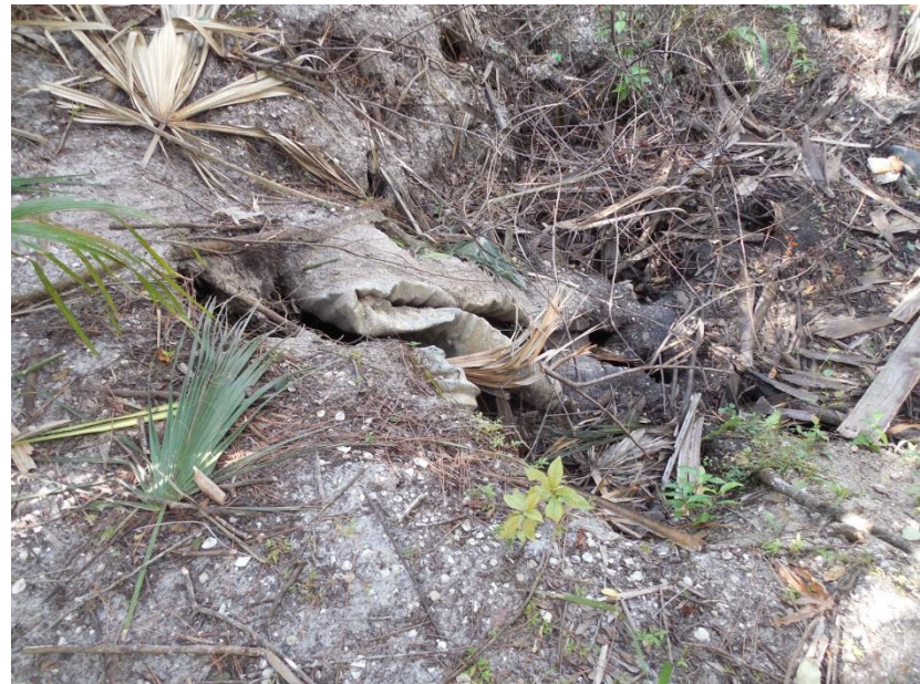
Mangled Dump Culvert
